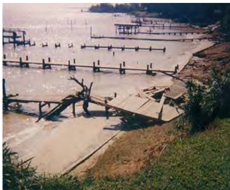
Storm damage incurred on the York River during Hurricane Isabel, 2003. Photo credit: J. Rickards.
